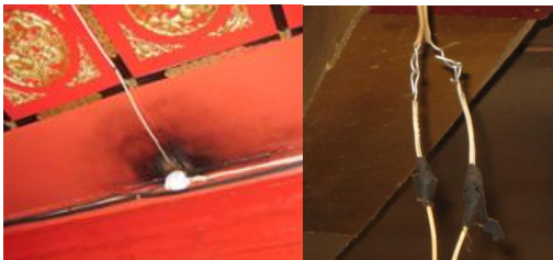
Electrical wiring issues and signs of overheating
